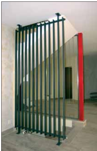
Figure 3. The radiator of the staircase is controlled by a KNX valve and also functions as a handrail.
